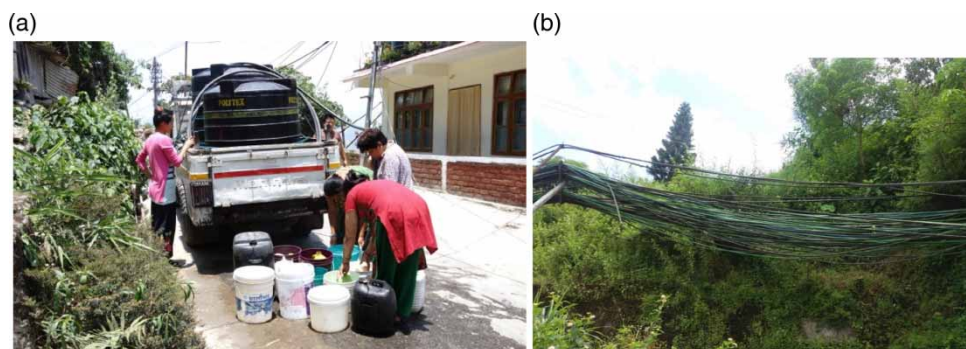
Fig. 7. (a) Water distributed by tankers at Kalimpong. (b) Supply pipes to Kalimpong, PHED's and privately owned.
