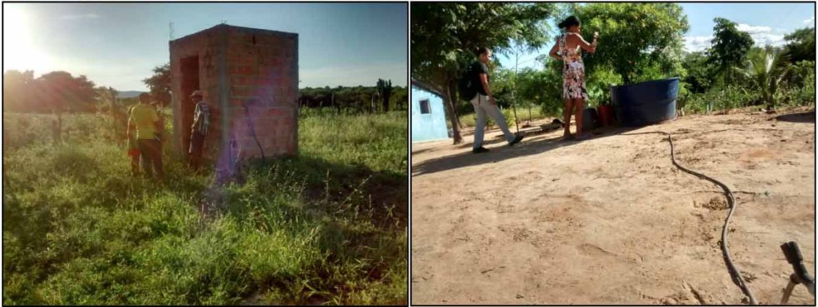
Fig. 7. Left, pump house built above the deep pit. On the right, a faucet installed in the backyard of one of the houses, to where the well water is pumped.
