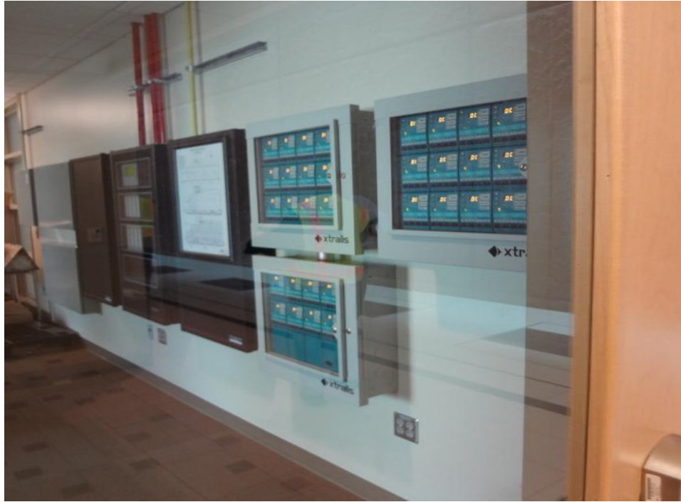
Nanofabrication cleanroom H5 Emergency Control Station, from 2013 Micro/Nano Edition.
