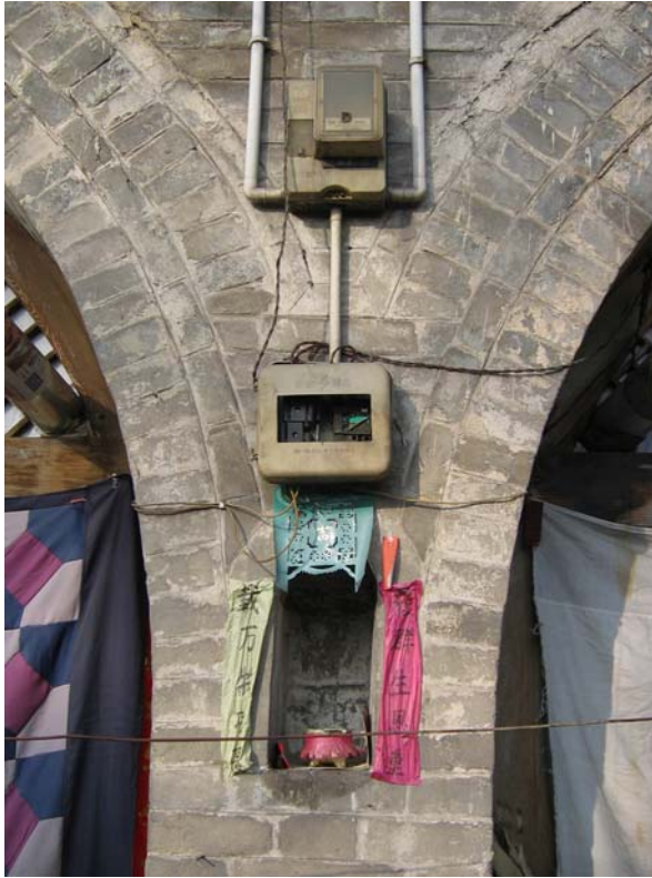
Fig. 3 In the most rural areas, electric switches and wires still look like in a spontaneous state of lacking security (source: Shaqu, Shanxi province, 2008. Photograph: Hu Xiaohui)
