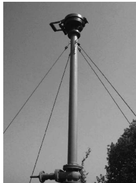
Figure 7 | A passive extraction well at the site.
