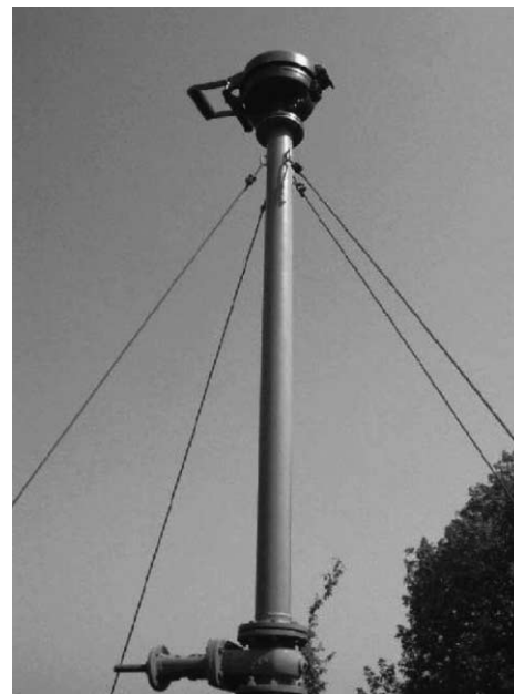
Figure 7 | A passive extraction well at the site.
