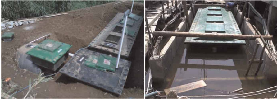
Figure 3 | Prefabricated DEWATS in Indonesia.
