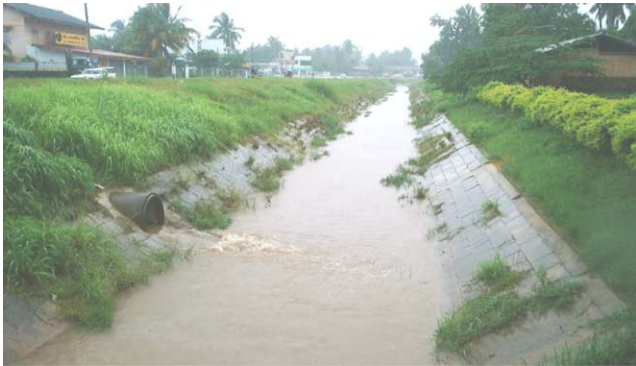
Figure 2 | Stormwater inlet to the Nam Pasak II, ca 1300m from the top (photo: Lacoursière & Vought, August 2001).
