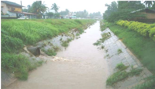
Figure 2 | Stormwater inlet to the Nam Pasak II, ca 1300m from the top (photo: Lacoursière & Vought, August 2001).
