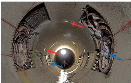
FIG. 2. The drift prepared for installation. The plugs fastening ring is casted in place approximately at the position of the camera. Some total pressure sensors are marked with red arrows and cable piping with blue arrows.
