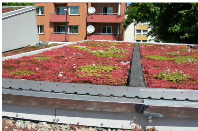
Figure 1 | Sections SD (from the left) and S0 of the extensive vegetated roof, Augustenborg, Malmö, Sweden.
