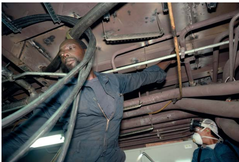
Fig. 2. Pipe fitters finishing the engine room of a tuna-fishing boat. Campbell Shipyard, San Diego harbor, August 1991. Originally published in Allan Sekula's Fish Story . Courtesy of the Allan Sekula Studio.
