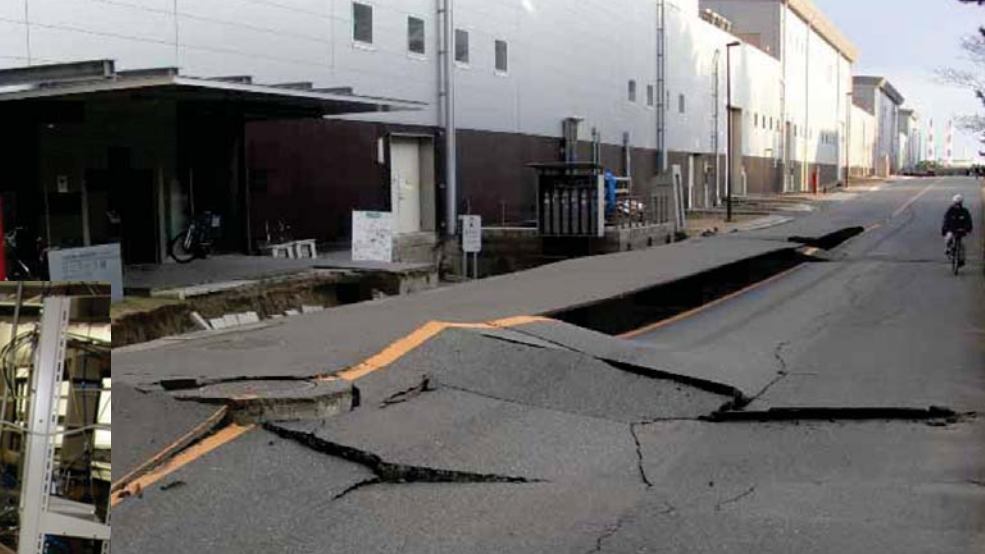
A cracked road running in front of the linac at the Japan Proton Accelerator Research Complex and a physics lab at Tohoku University are examples of damage wreaked last March by the 9.0-magnitude Great East Japan Earthquake.
