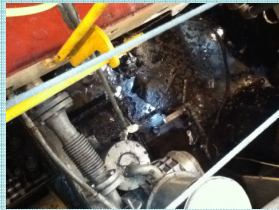
Oiled Engine Room prior to use of solidifier
