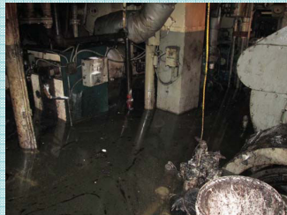
Condition of engine room with improved visibility after use of solidifier granules.
