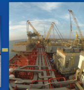
Both MCVs arrived in Gulf of Mexico for integration and commission testing
