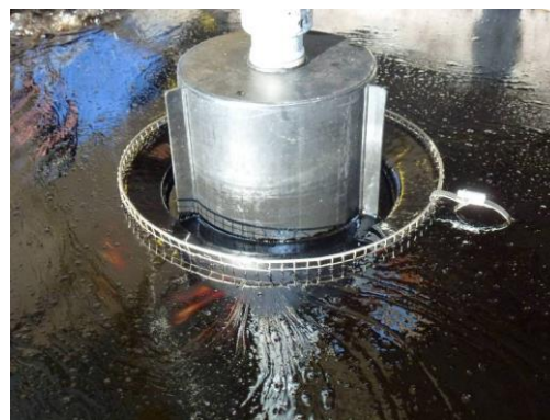
FIGURE 6. MECHANICAL SELF-ADJUSTING WEIR SKIMMER IN OPERATION.
