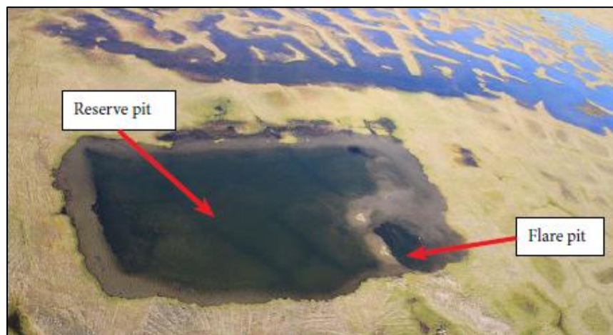
Figure 8: An aerial photo of South Simpson #1, showing the collapsed berm between the flare and reserve pits (US BLM, 2013).
