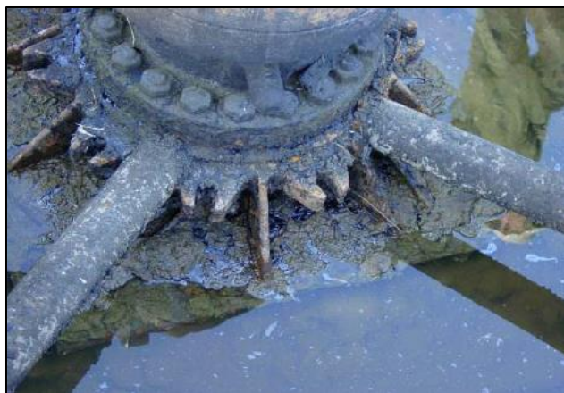
Figure 7: Visible sheening from within the Fish Creek #1 well cellar (US BLM, 2013)
