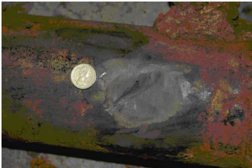
Figure 1 | Typical surface condition of supplied cast iron pipe showing extensive graphitic corrosion of pipe wall.
