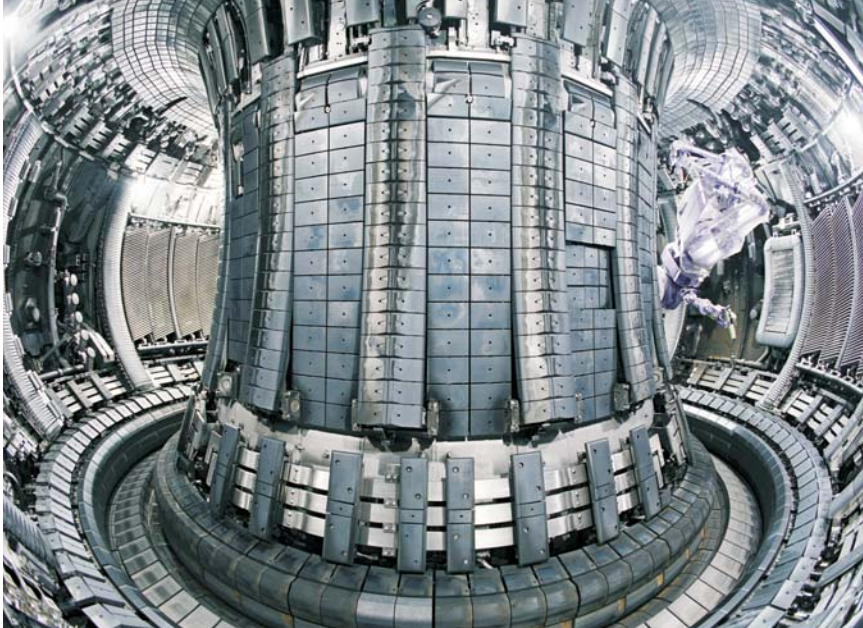
The thousands of carbon tiles lining the plasma-facing wall inside the vacuum vessel of the Joint European Torus are being replaced using a remote-controlled slave arm.
