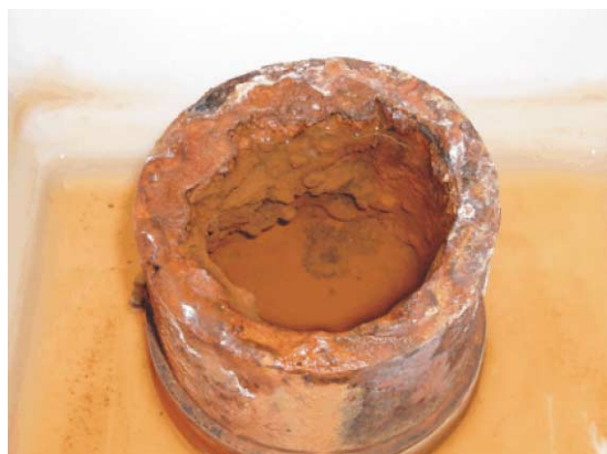
Figure 1 | Photograph of 4 inch diameter cast-iron pipe section used in study.
