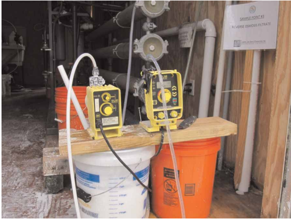
Figure 1 | Lime slurry feed pump and bucket (white on left).
