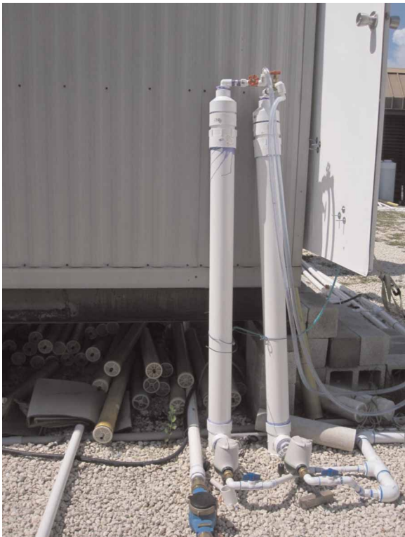
Figure 3 | Lime and kiln dust filters.
