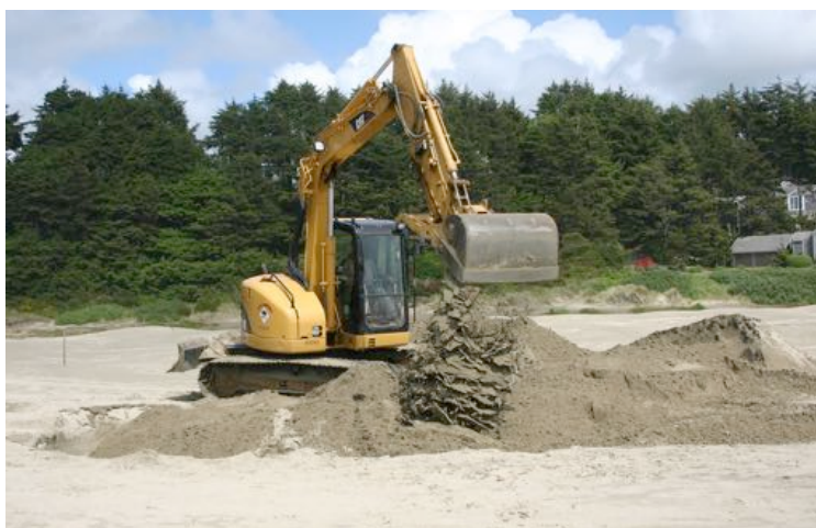
Figure 7. The excavator fills the hole back in with sand. Photo: Oregon Parks and Recreation Department.
