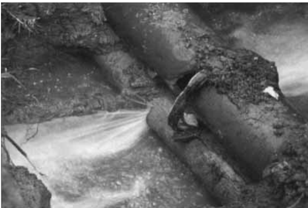
Figure 4 | Leaky water pipe laid next to a sewer pipe (source: Gary Feeny, Earth Tech. Reprinted from Opflow 25(9), September 1999 by permission. Copyright © 1999, American Water Works Association).
