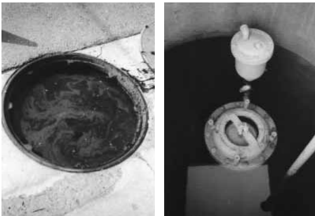
Figure 2 | Submerged air release valve.
