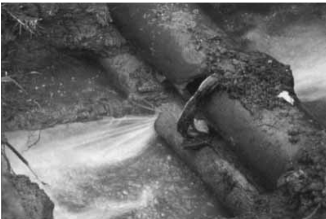
Figure 4 | Leaky water pipe laid next to a sewer pipe (source: Gary Feeny, Earth Tech. Reprinted from Opflow 25(9), September 1999 by permission. Copyright © 1999, American Water Works Association).
