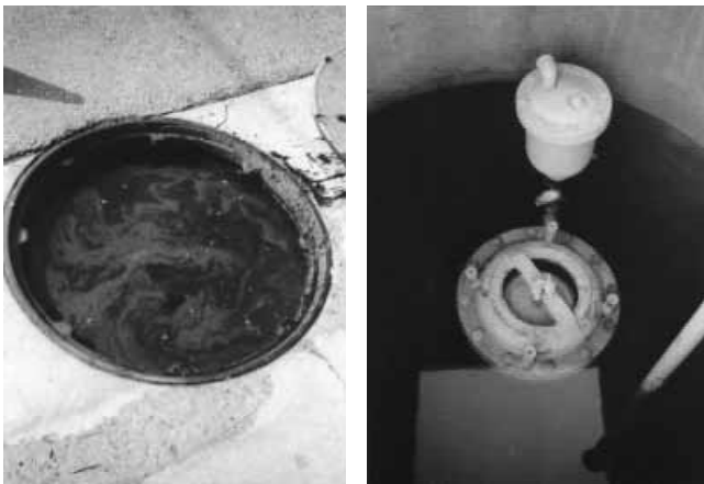
Figure 2 | Submerged air release valve.
