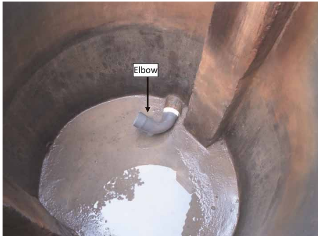
Figure 5 | Aeration tank with elbow installed.
