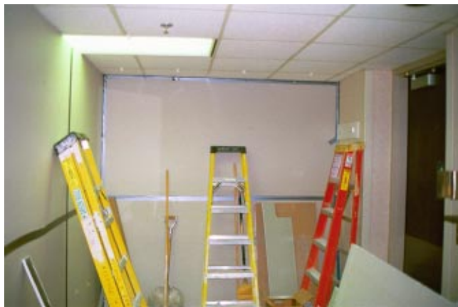
Fig. 3 Photograph of the construction side of a barrier in a hospital corridor separating the construction zone from the occupied area (Source: Richard Hermans, Center for Energy and Environment, Minneapolis, MN)
