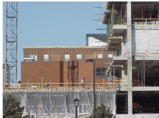
Fig. 1 Photograph of new construction in front of a 1970's hospital building with mechanical ventilation that was added to a 1920's building originally designed for natural ventilation with operable windows.
