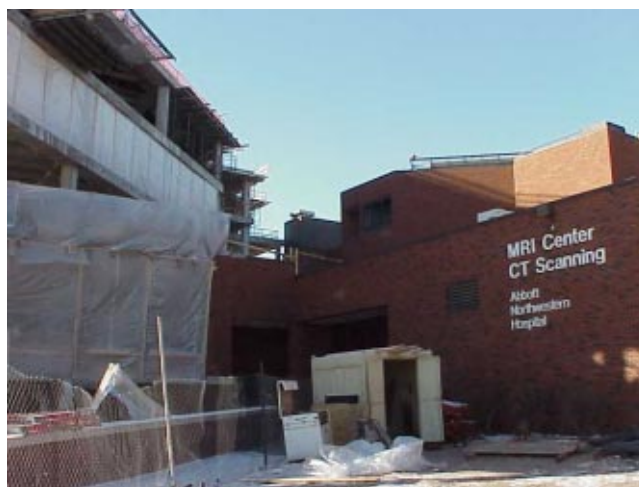
Fig. 2 Photograph showing new construction of a large heart center connected to an existing hospital building near the MRI/CT Scanning unit
