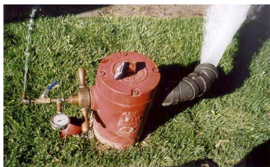
Figure 2 | Sampling device installed on the fire hydrants.
