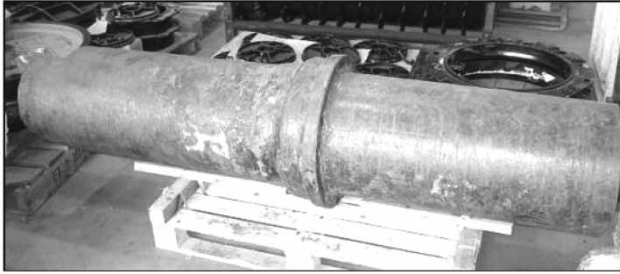
Figure 1 | The outside surface of cast iron for water supply pipe constructed in 1887 in Yokohama City.
