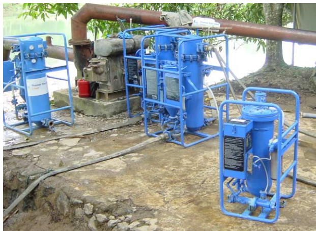
Figure 3 | Stella Meta Pre-Coat Filters in Operation in Aceh.
