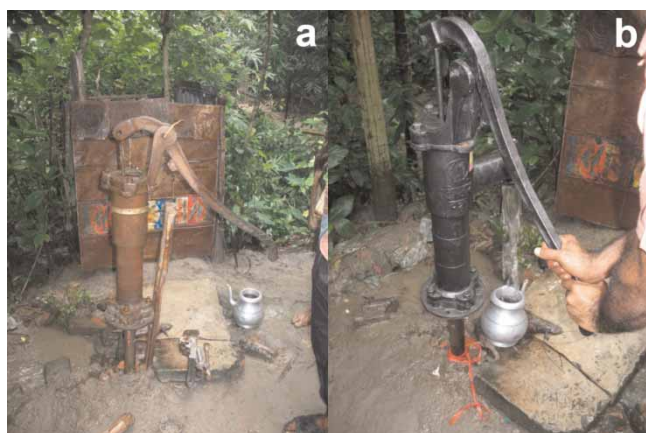
Figure 1 | Tubewell no. 21602 (a) with original hand-pump attached and (b) replaced with a new hand-pump.
