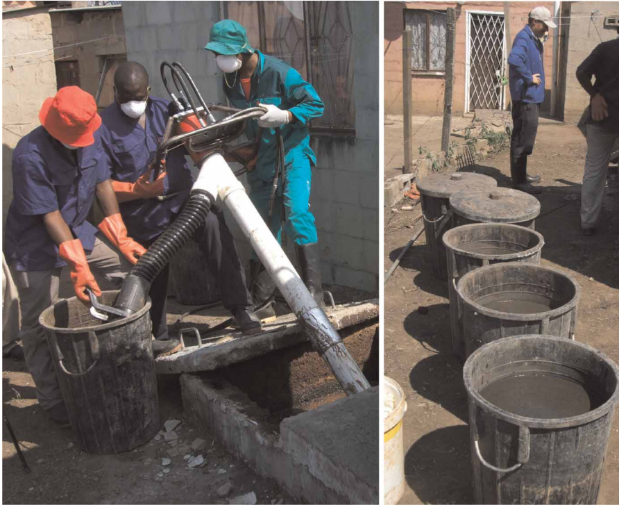
Figure 5 | Extraction auger being used to empty pit latrine in Durban, South Africa.
