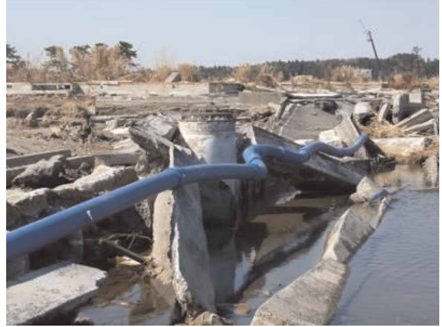
Figure 3 | Damage to pipe by tsunami-induced scouring.
