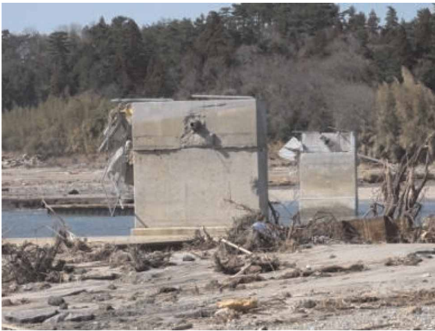
Figure 2 | Washed-away water pipe bridge.
