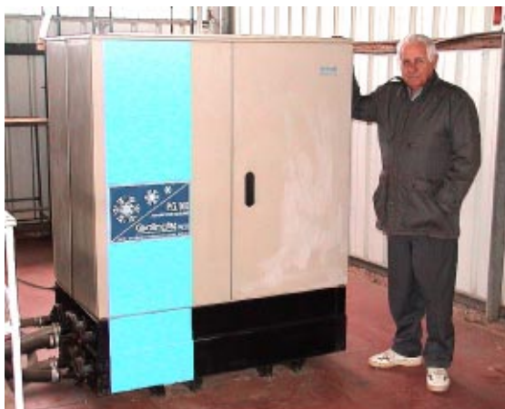
Fig. 12 The Coolingtec absorption-cooling machine
