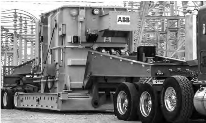
1.4 Outages are not just overnight when major equipment fails: a RecX “spare tire” recovery transformer arrives at a substation. Courtesy of ABB.
