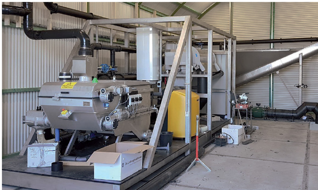
Figure 8.3 An RBF system is demonstrated at the sewage treatment plant of Geestmerambacht (The Netherlands).
