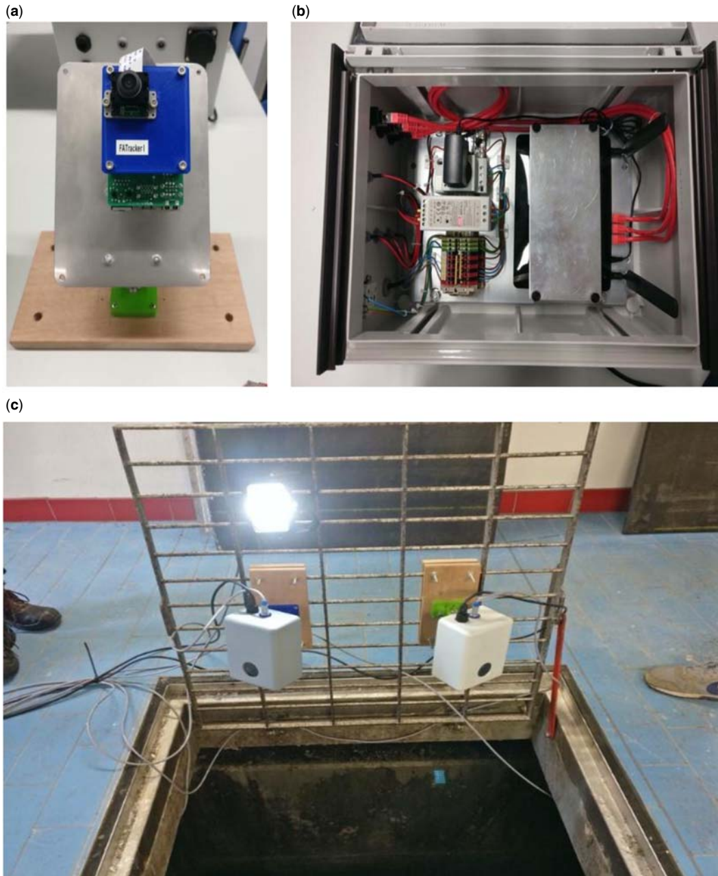
Figure 6.19 Example of cameras installed in a wastewater pumping station: (a) Camera including electronics; (b) Camera housing, (c) Two cameras installed at a grate in a wastewater pumping station. Source: courtesy Antonio Moreno-Rodenas (Deltares).
