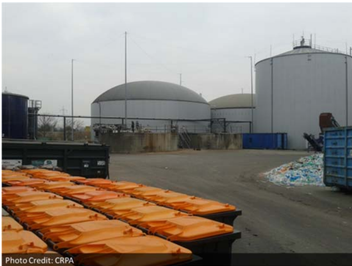
Figure 6.2 Waste biogas plant.
