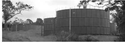
Figure 4.7 A few of the larger potable water storage tanks for Kilauea Military Recreational Camp.
