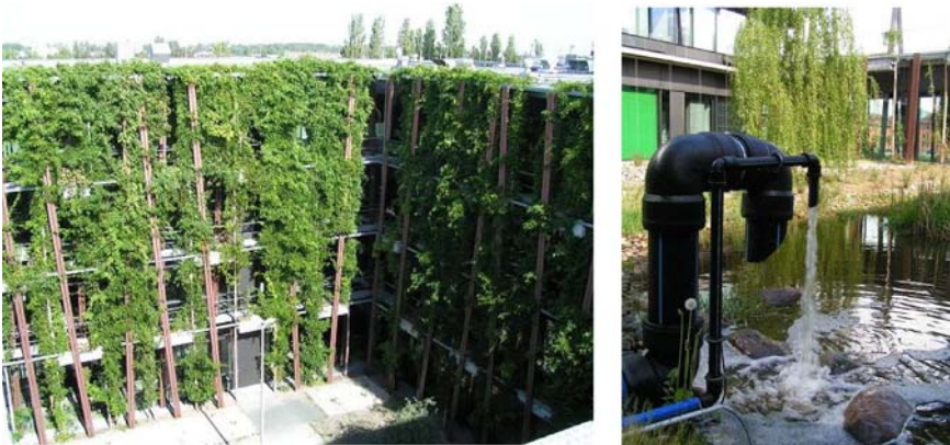
Figure 17.5 Façade greening system (left), artificial rainwater pond combined with trough infiltration for stormwater management (right). (Source: Author's own).
