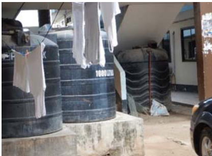
Figure 18.15 PVC tanks in Dar Es Salaam. (Source: Author's own).
