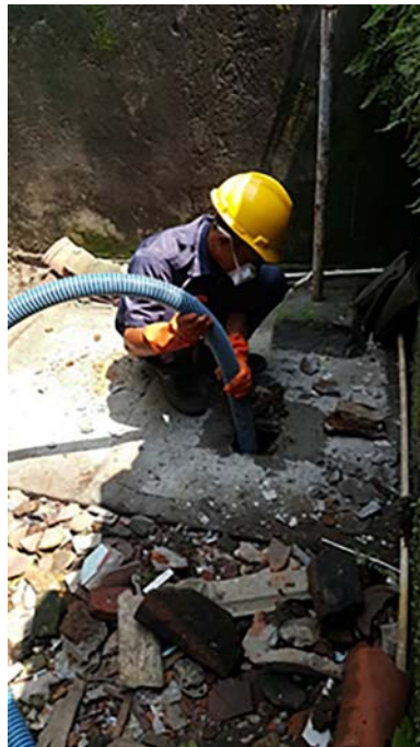
Figure 0.3 The City of Surakarta (Central Java) has implemented the scheduled desludging scheme as required by the local regulations. Each septic tank must be desludged every 3 years. The local water supply firm is appointed to manage the scheduled desludging in 2015.
