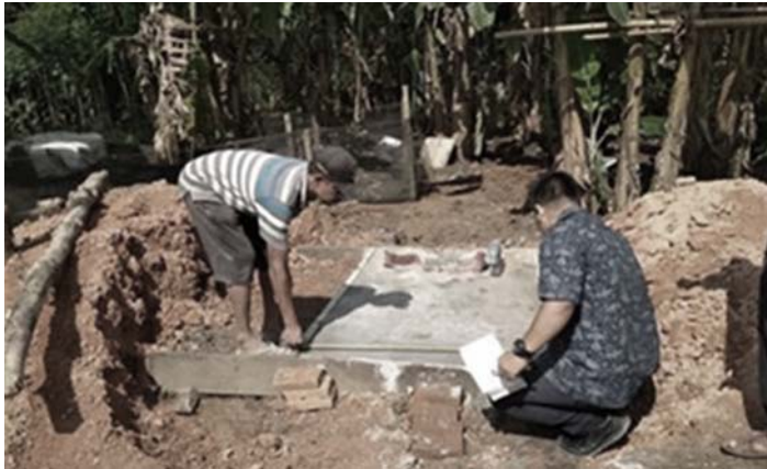
Figure 8.4 The municipality needs to regularly inspect every septic tank in its area, particularly to find out the condition, the utilization and the last desludging conducted. It is also necessary for the municipality to check on under-construction septic tanks.
