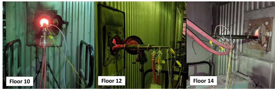
Fig. 1 Images of University of Utah narrow-angle radiometer setup at each boiler elevation examined
