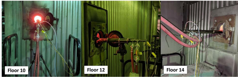
Fig. 1 Images of University of Utah narrow-angle radiometer setup at each boiler elevation examined
